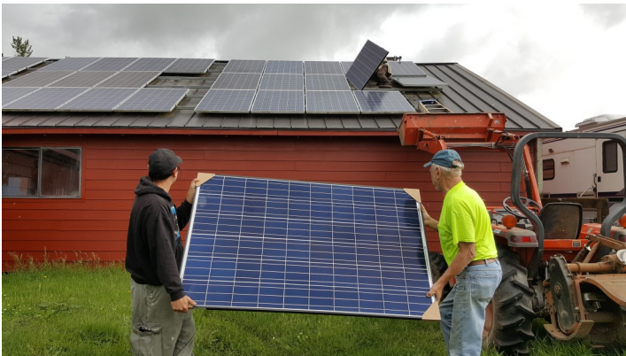
Our crew, Nils and Ken Dunder, carrying new panel for mount on roof.
