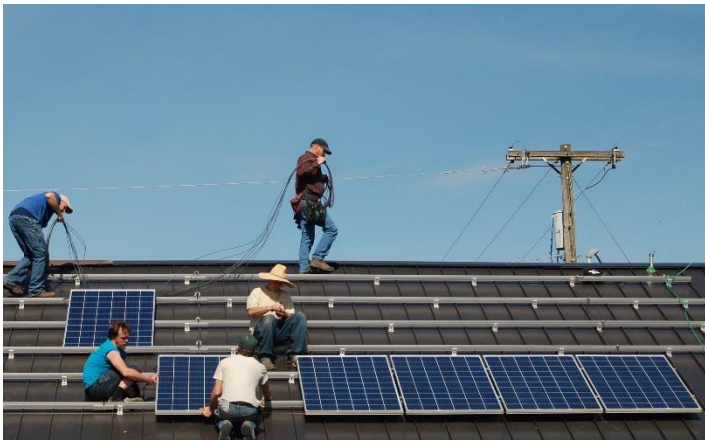
Solar modules are installed and electrical lines are hooked up linking the modules and Fronius inverter.
