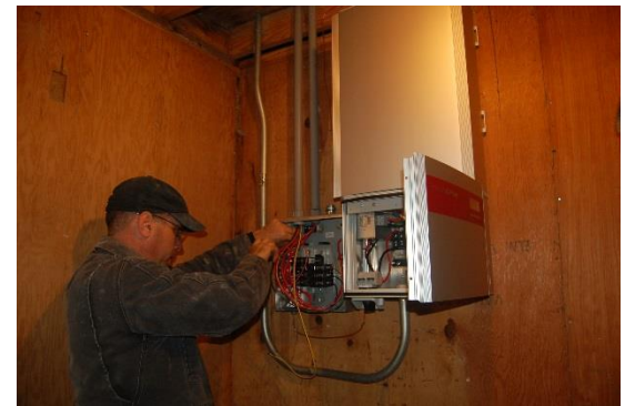
Electricians install Fronius inverter and AC/DC disconnect and 400/320A 200 dual feed service to PGE..
