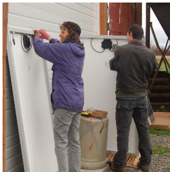
Laura and her crew prepare solar modules for mounting on the roof racks.
