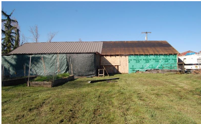
Equipment barn: right side of roof was removed and interlocking metal roofing was installed.
