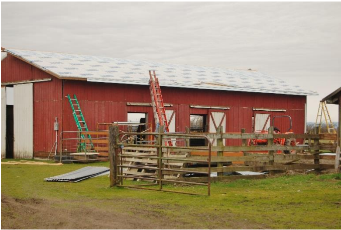
Horse barn: The metal roof was removed. Ken, Luke and Phil installed OSB board and extended the roof, allowing soffits and gable. Tyvek was added. Metal roof taken from the equipment barn was moved and installed onto the horse barn. The balance of the metal roof from the horse barn was reused and extended with add-ons to accommodate the added width of the roof.
