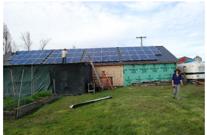
12,480 W system installed, again allowing space for maintenance and cleaning of the solar modules.
