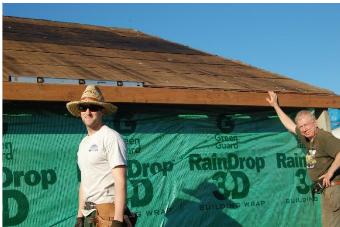
Our son, Luke Fitzpatrick, helped with all aspects of the project. Luke and Ken install OSB board and soffits.
