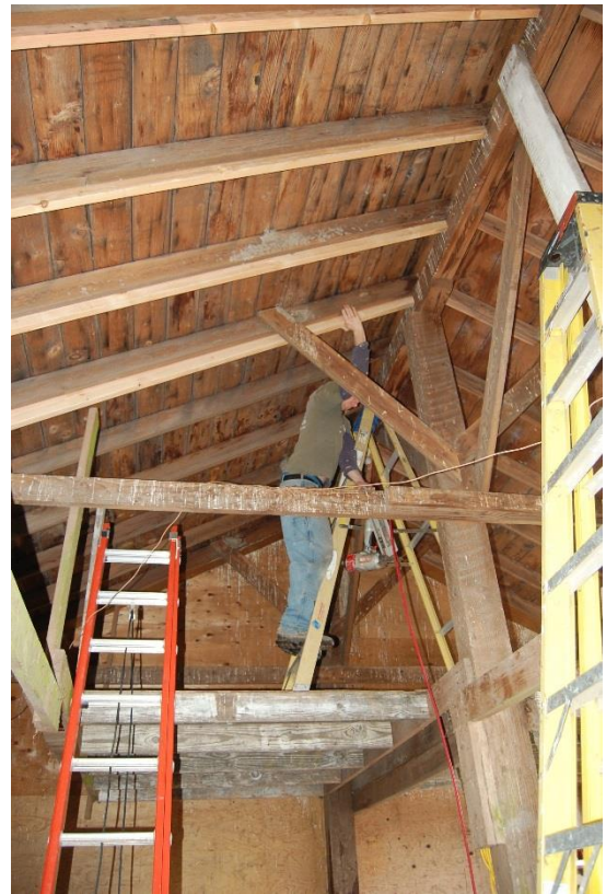
Interior of equipment barn. 2X6's added widthwise on the barn roof (above and right).
