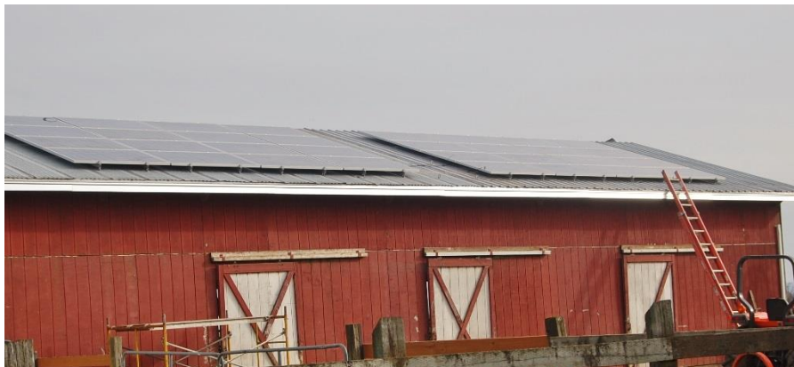
Completed installation on the horse barn. 7920 W system, with ample room provided to maintain and clean the solar panels.
