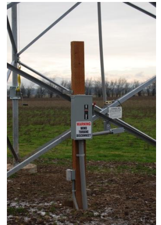
Electrical turn off at turbine.
