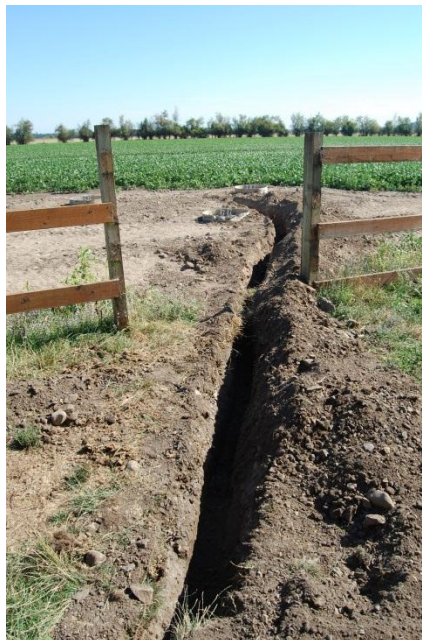
Underground line to turbine.
